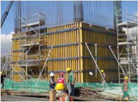
DATA CENTER BANCOMER
